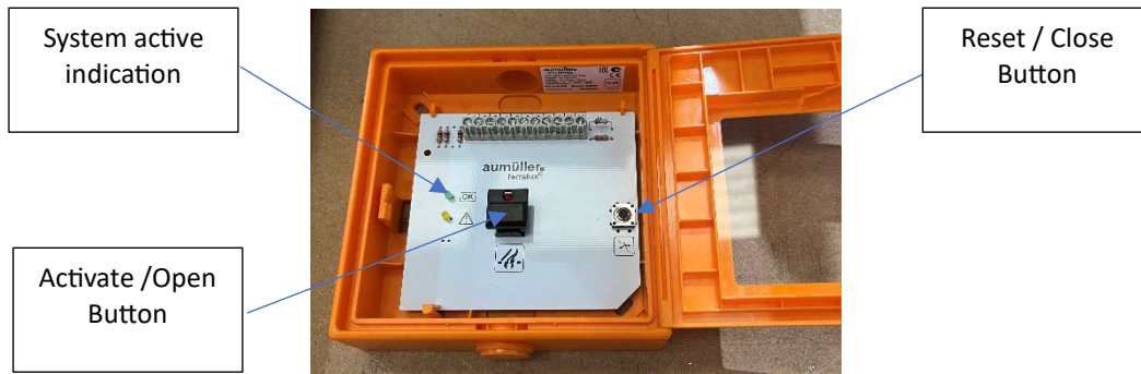
Picture 2 – Manual Call Point (aka Breakglass Unit)
