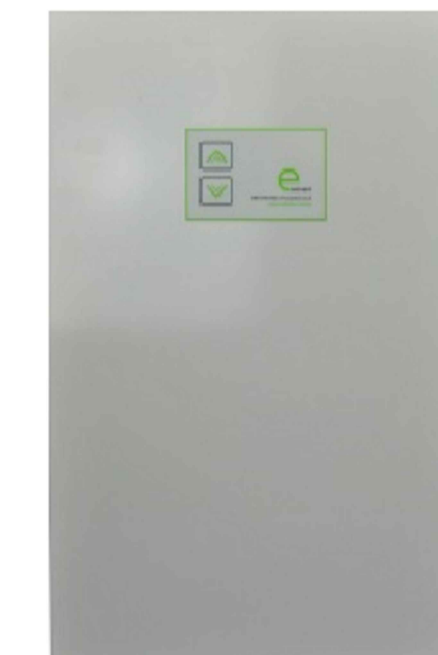
VENT 6 CONTROL PANEL
